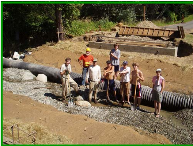
Volunteers assist the contractor with restoring the site before the bridge slabs are installed.
