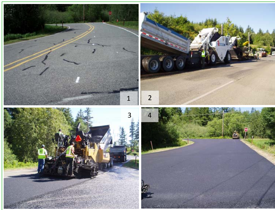
1. Sealed cracks in the existing pavement at the Eaglemount Road intersection with Center Road are visible indicators of distressed pavement. 2. Lakeside’s paving equipment train ready to begin paving. It took three days for Lakeside to pave the 2.4-mile-long project. 3. A 2-in asphalt mat was overlaid on top of existing pavement. 4. Compaction testing results on Center Road exceeded minimum standards, ensuring the longevity of the new pavement.
