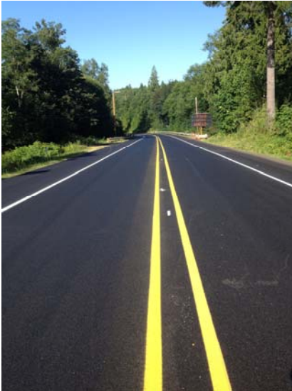
The newly rehabilitated asphalt surface and striping on Center Road provides an improved ride quality.
