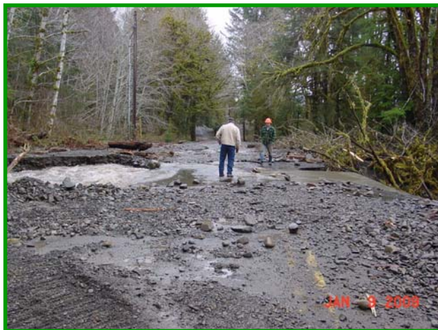
After the storm event in January, 2009, debris covered the Upper Hoh Rd and water eroded parts of the road surface.
