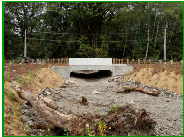
The new box culvert is 22-ft wide and 40-ft long. Other improvements to Spruce Creek included grade controls to improve streambed stability and protect the structure from scour.
