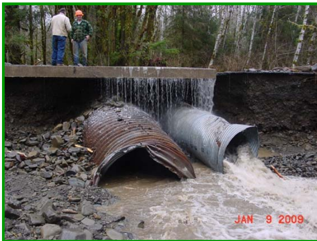
The old Spruce Creek culverts—with diameters of 72-in and 48-in — and the Upper Hoh Rd above, damaged by flooding.
