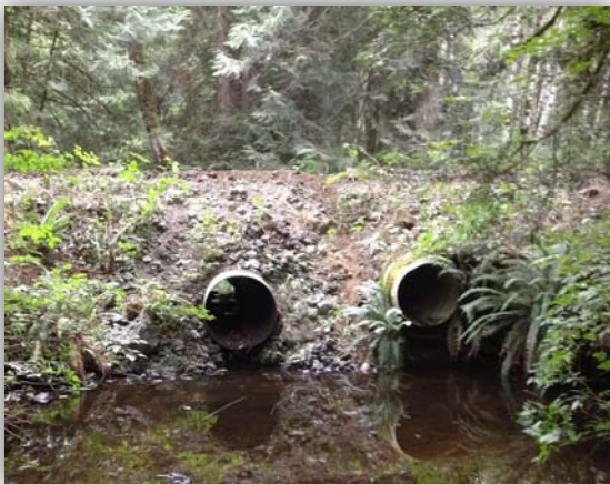
The two, old culverts on Andrews Creek were barriers to fish passage and were in poor condition.
