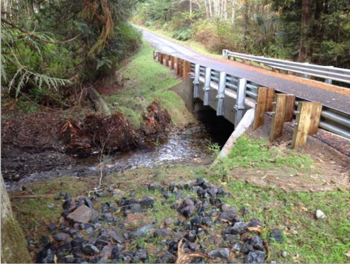
The newly, reconstructed Snow Creek Road, with a view of Andrews Creek flowing along the reconstructed creek bed.
