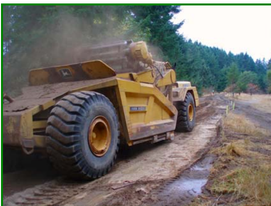
Project construction activities adjacent to the trailhead (shown above) and along the trail route included clearing and grading, applying new surfacing and installing fences.
