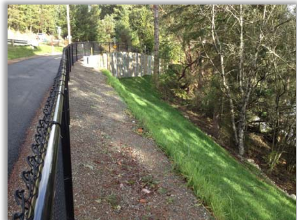
A soldier pile wall was constructed along a steep grade to allow room for the trail.
