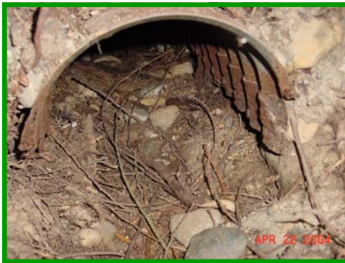
The existing cross culvert under the road at MP 8.947 was badly deteriorated.
