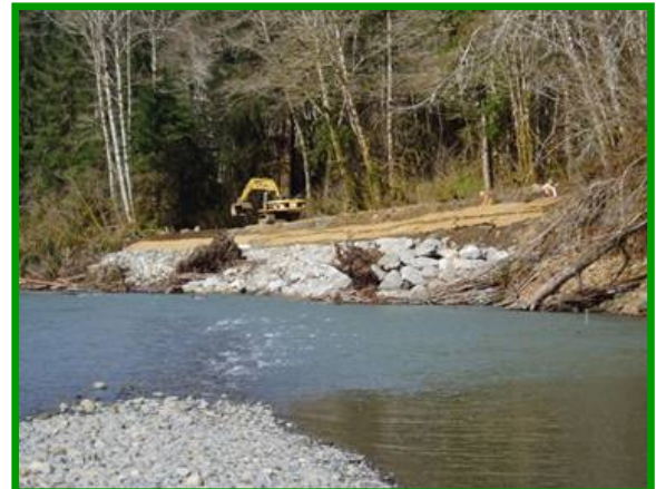
The erosion control blanket will biodegrade over time and willow roots will form a dense mat that will help to hold the embankment in place.
