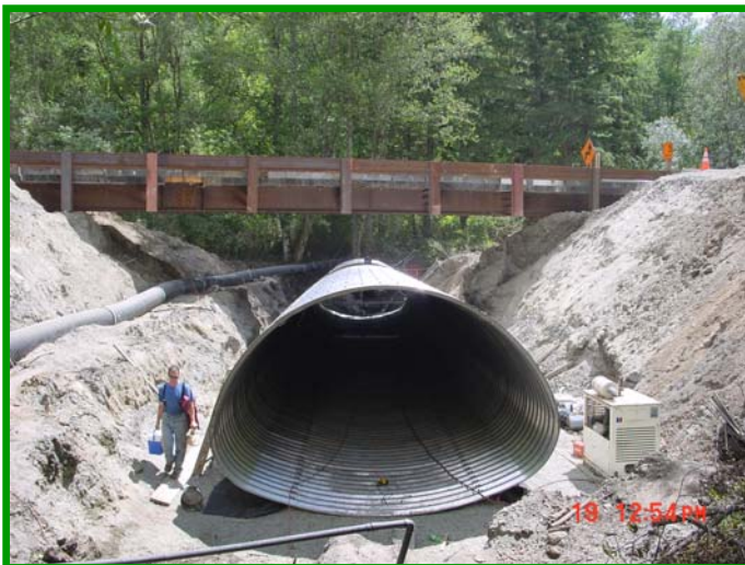
The culvert project at Center Rd required a temporary bridge to handle traffic during construction.
