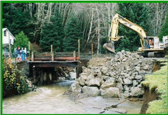
Damage to the old Fossil Creek Bridge occurred in 2003.
