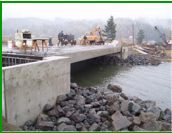
During construction of the new bridge, a temporary one-lane bridge was installed for through traffic.
