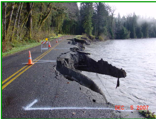
High river flows in December, 2007 washed away a portion of the Upper Hoh Road at milepost 7.8.
