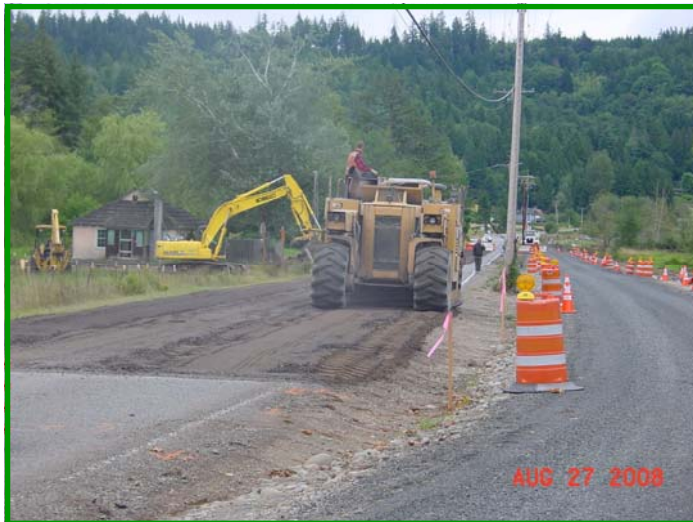
During East Quilcene Rd reconstruction, a temporary bypass (shown on the right in the photo above) was opened to accommodate thru traffic while work continued on the road.
