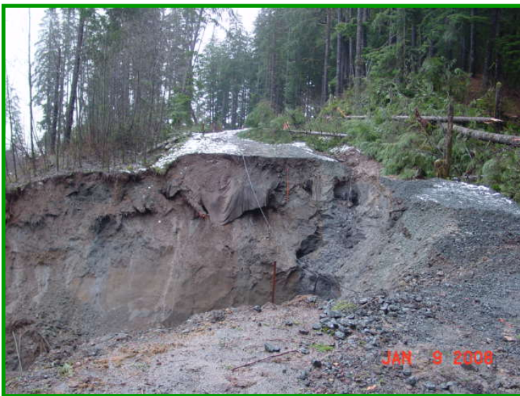
This image, taken January 9, 2008, shows Dowans Creek Rd after high water flows in the Bogachiel River caused slope failure and washed out the road.
