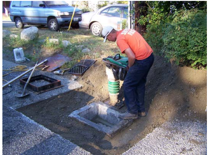
▲ Improving drainage was an important component of this project. In this photo, Corey Woodley compacts backfill material around a new catch basin.
