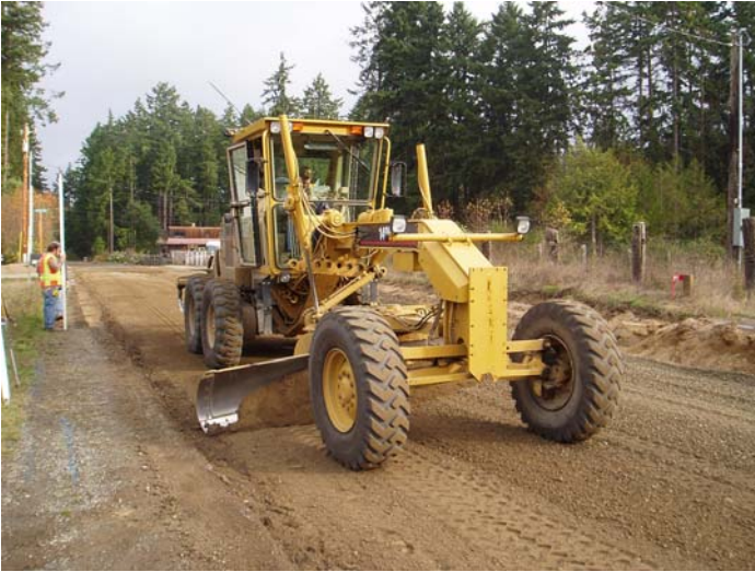
▲ Building a great road means constructing the foundation just right. Equipment Operator Rock Fountain grades road base material while road superintendent Paul Walters checks grades.
