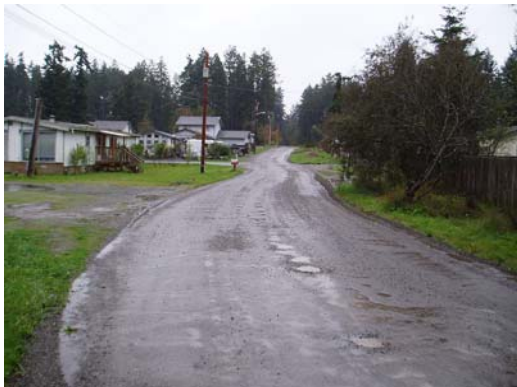
Before improvements on 6th Ave, the uneven gravel surface, dust, potholes, and poor drainage were problematic.
