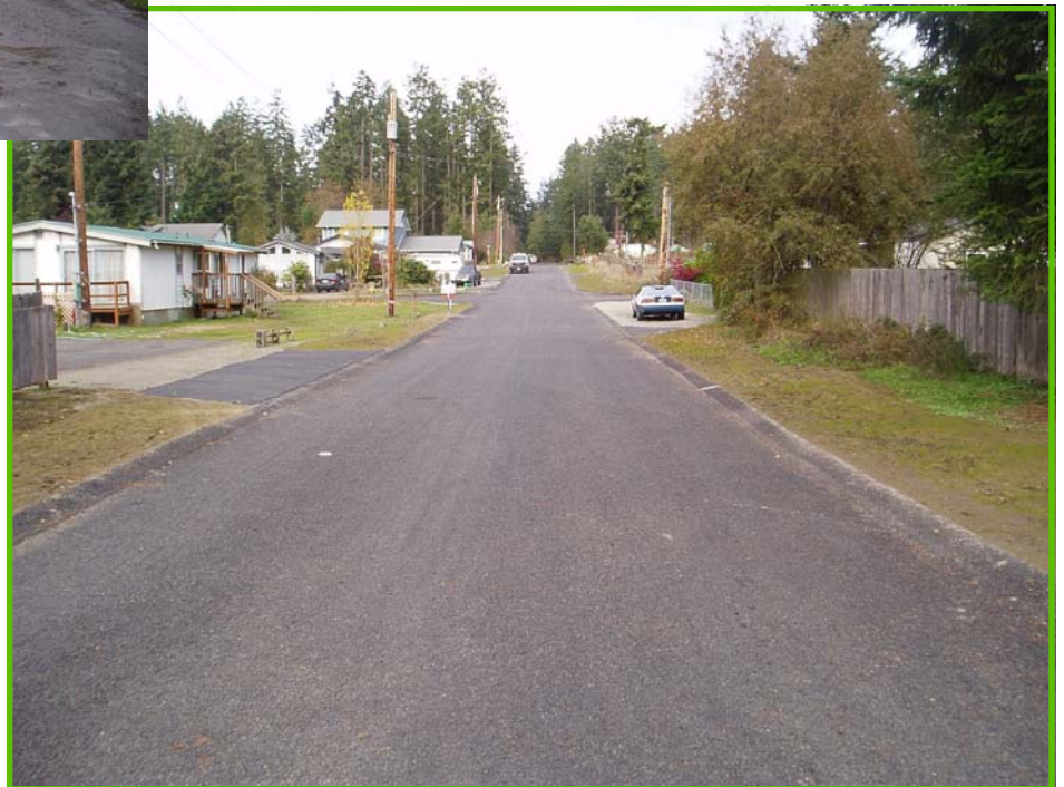
The upgraded 6th Ave: Horizontal re-alignment, the new chipsealed surface and drainage structures are a great addition to the neighborhood.
