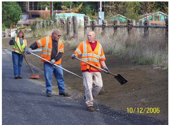
▲ A project is not complete until the area impacted by construction is groomed and landscaped. Larry Taylor and Larry Guenther smooth top soil along the roadside while Crystal Moore sweeps excess dirt off the new pavement.
