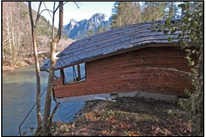
House damaged by Skykomish River flooding.
