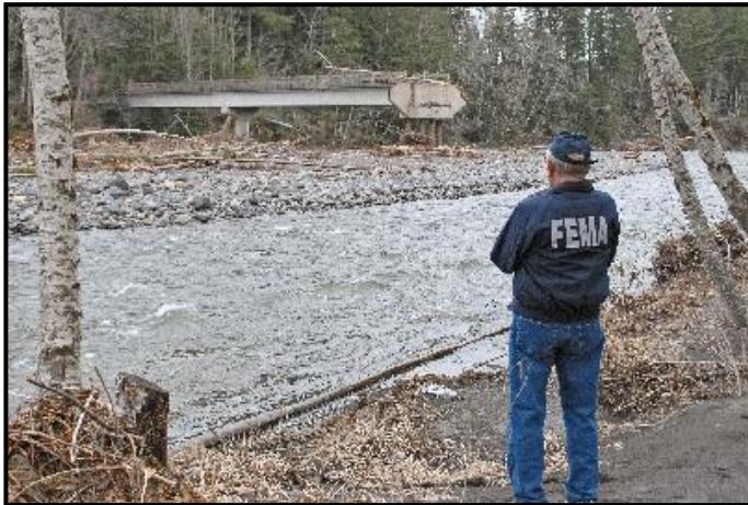
FEMA official inspects flood damage to a bridge.
