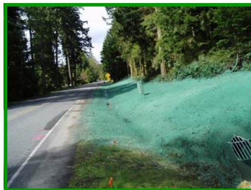
Final work included hydroseeding the construction area. The outlet of the new stormwater system is visible on the right.
