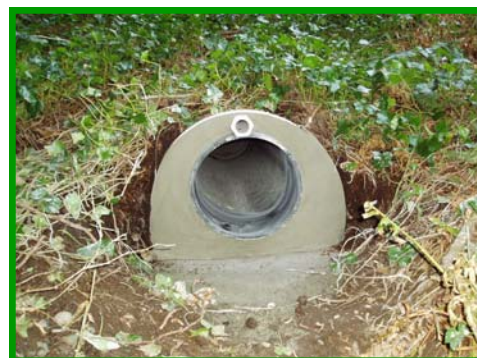
The newly installed, 'sliplined' culvert. The space between the two pipes is filled with grout and the ends sealed.
