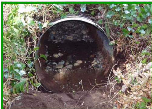
The original 36" diameter culvert under the road at MP 9.066 was badly deteriorated.
